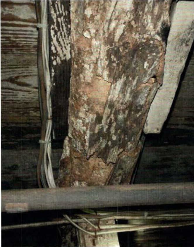
Photo S: Damaged first floor girder in Basement C
