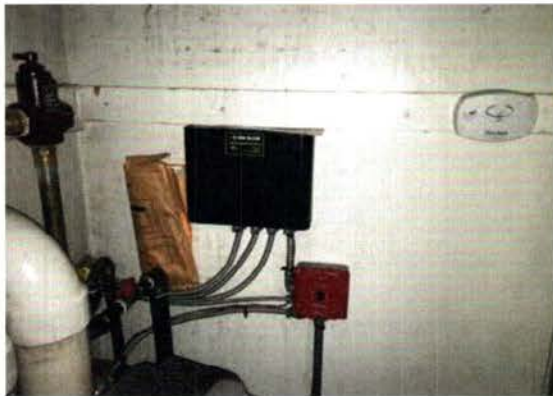
Fig. H-3 Boiler Controller & Shut Off (103A)
