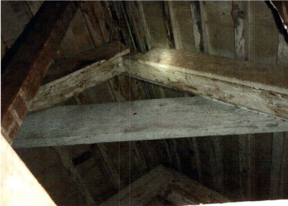
Photo H: Roof framing at original structure above Living Room (204A) and Bedroom #5 (204)
