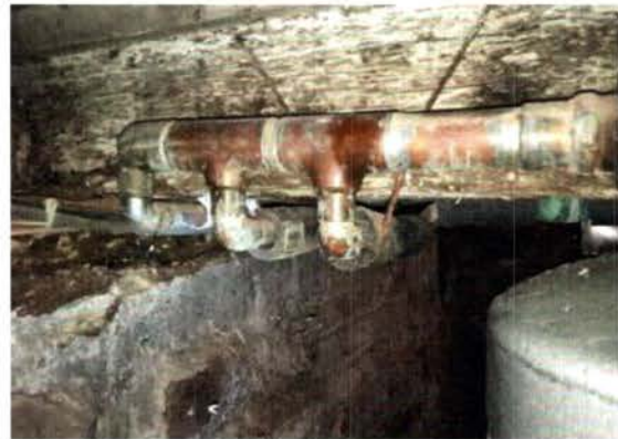
Fig. H-12 Close Up Of Uninsulated Piping And Wire Supports (002)
