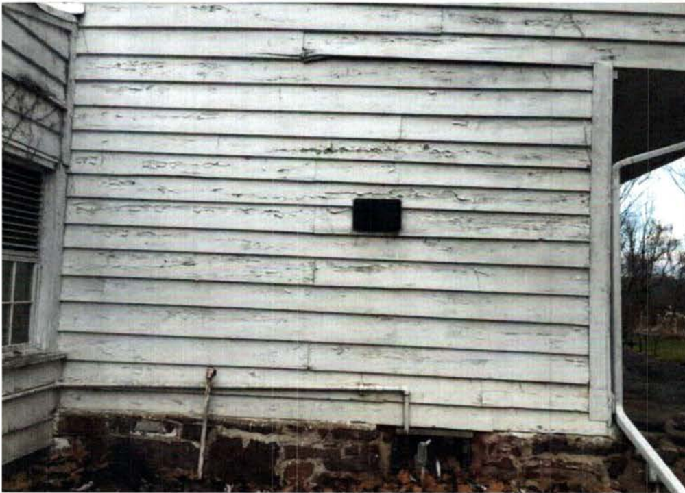
Fig. P-10- Exterior Roof Leader and Gas Piping
