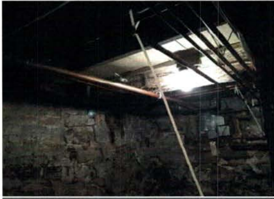
Fig. H-9 Heating Hot Water Uninsulated Piping (002)
