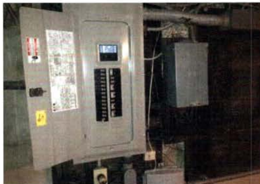
Figure E-5 Main House Wiringn (007)
