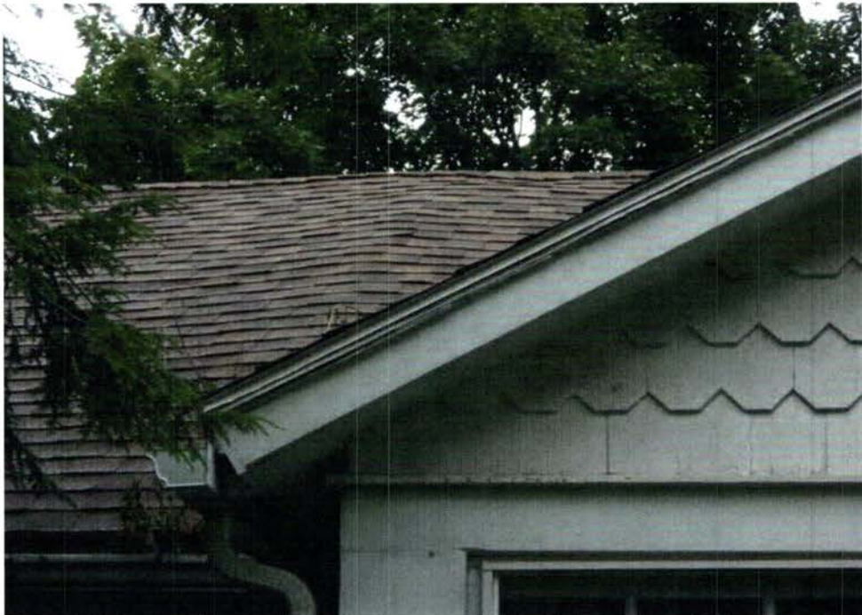
Photo E: Roof at the intersection of the center addition and the kitchen addition.
