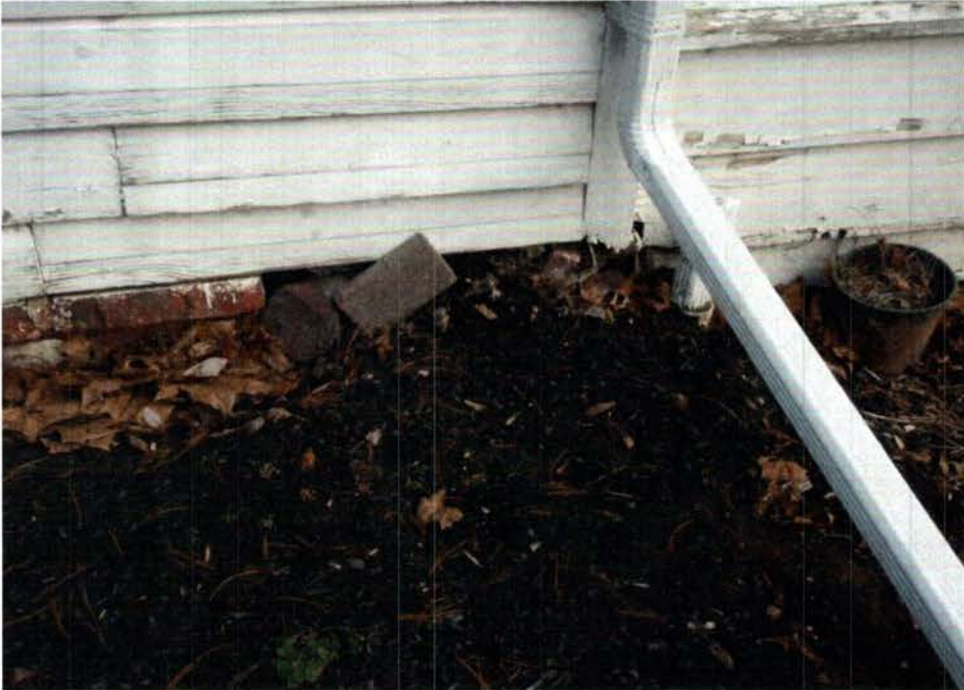
Photo G: Foundation deterioration at SW corner of original structure
