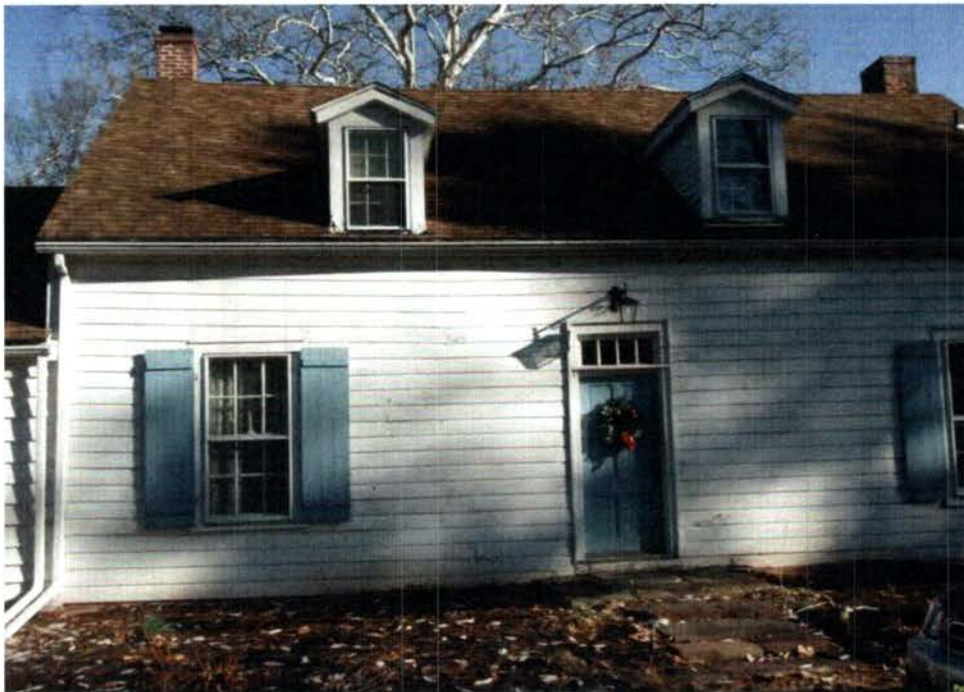
Photo B: West side of house in area of shifted siding and sagging roof
