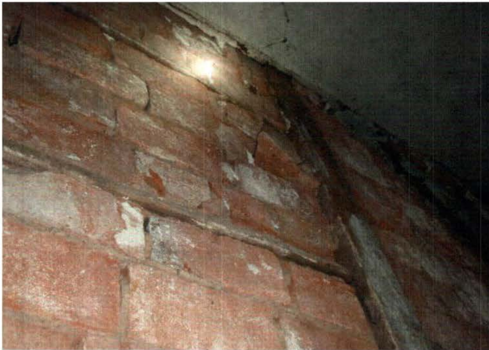
Photo J: Damaged brick at north wall of the center addition as seen from the kitchen stairwell to the basement.
