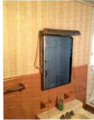
Figure E-8 Main Bathroom Mirror Receptacle (105)
