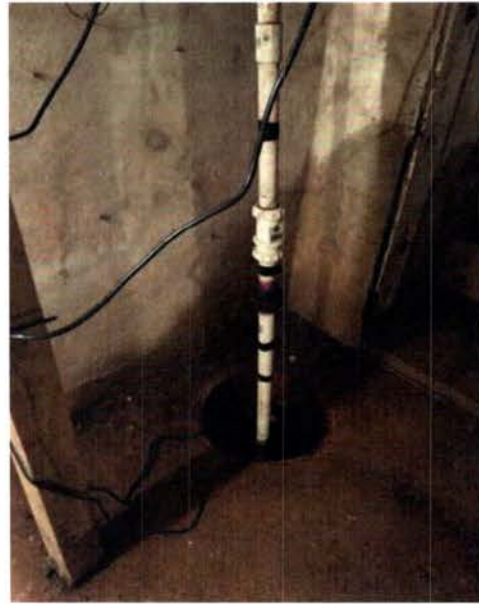
Fig. P-2-Simplex Sump Pump Located in Basement (007)
