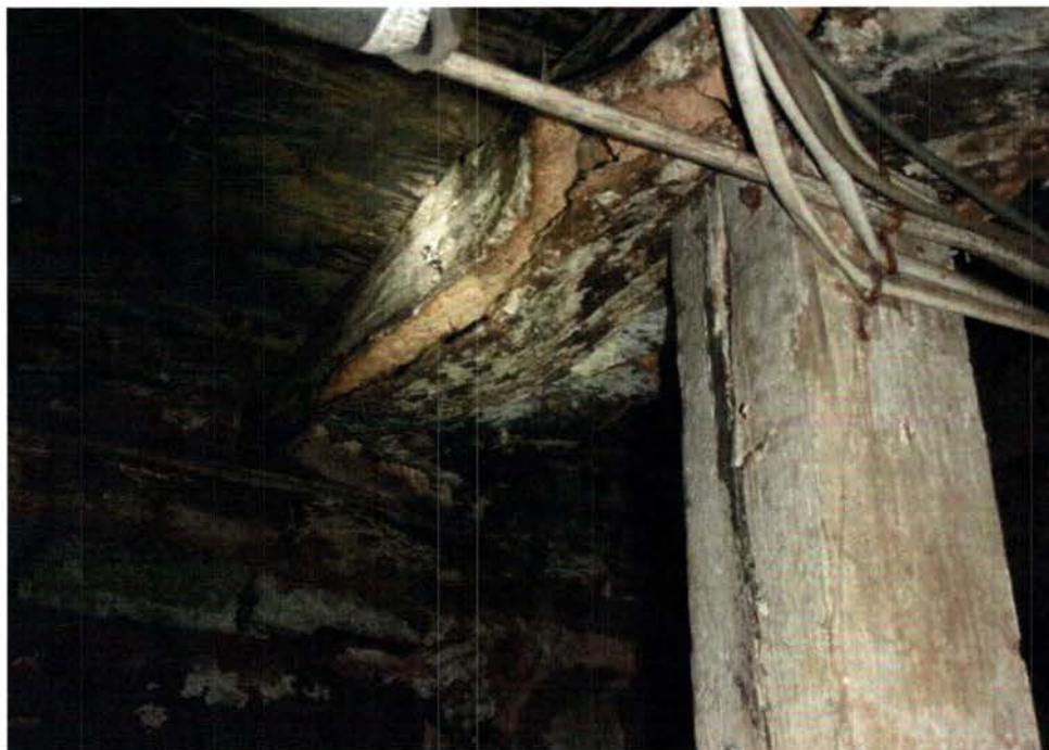
Photo R: Damaged first floor girder in Basement C
