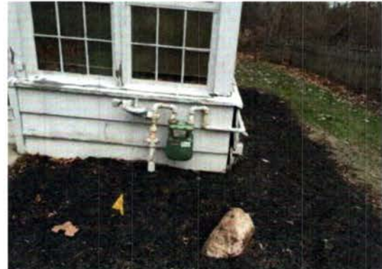
Fig. P-4- Gas Meter with exposed piping on exterior wall.
