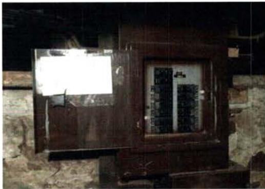
Figure E-3 Main House Sub Panel(003)
