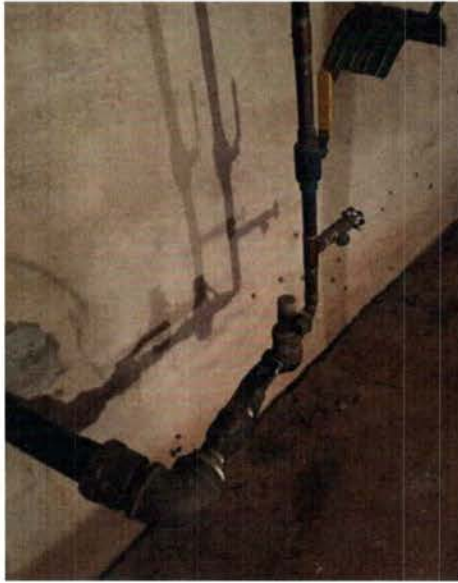
Fig. P-1- Domestic Water Main Entering Basement (007)
