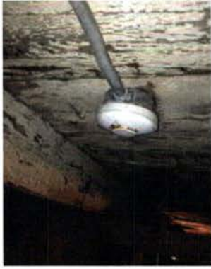
Figure E-19 Rusted Heat Detector (001)
