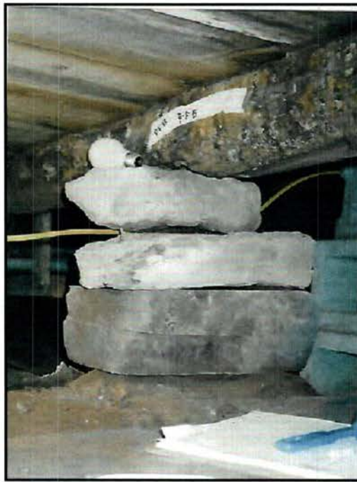
Plate 4.3: Undated photo showing a pier and floor joist within the crawl space. Note the masking tape label on the timber.
