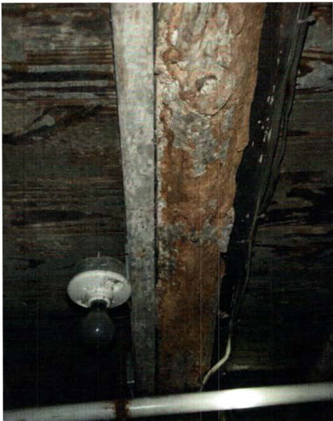
Photo Q: Damaged first floor girder in Basement C
