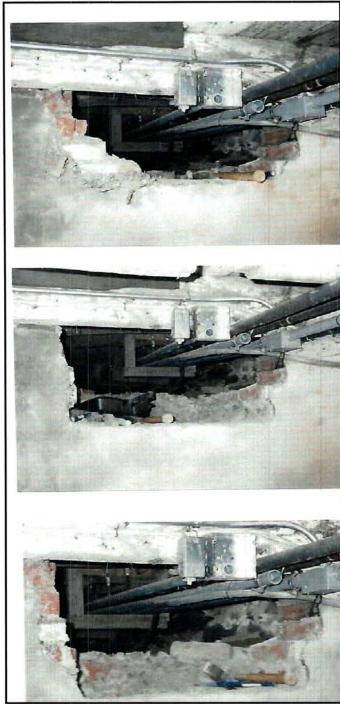
Plate 4.1: A sequence of photos showing the work done to enlarge the entrance into the crawlspace under the western addition of the house. View south.
