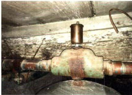
Fig. H-11 Close Up Of Air Separator (002)
