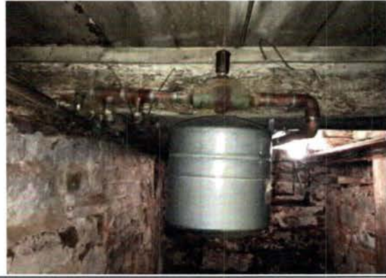
Fig. H-10 Air Separator And Uninsulated Zone Piping (002)
