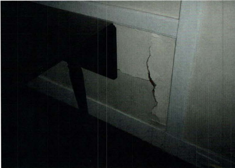
Photo K: Damage to the north wall of the center addition caused by water infiltration at the brick wall.
