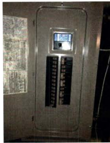
Figure E-2 Main House Main Electrical Panel (007)
