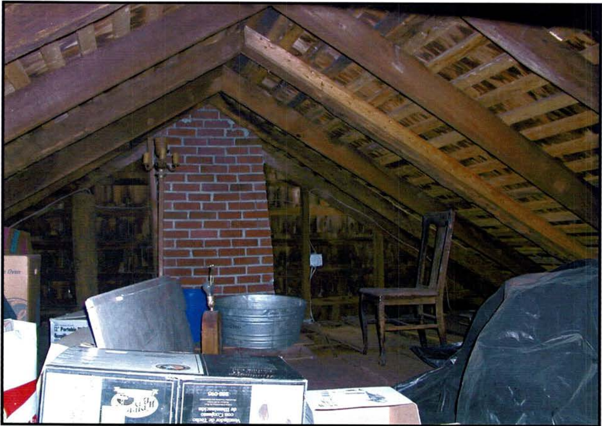
Attic of south (older) wing, showing sistered framing and re-used hand-hewn rafters. The chimney at the far end of the space was recently rebuilt.
