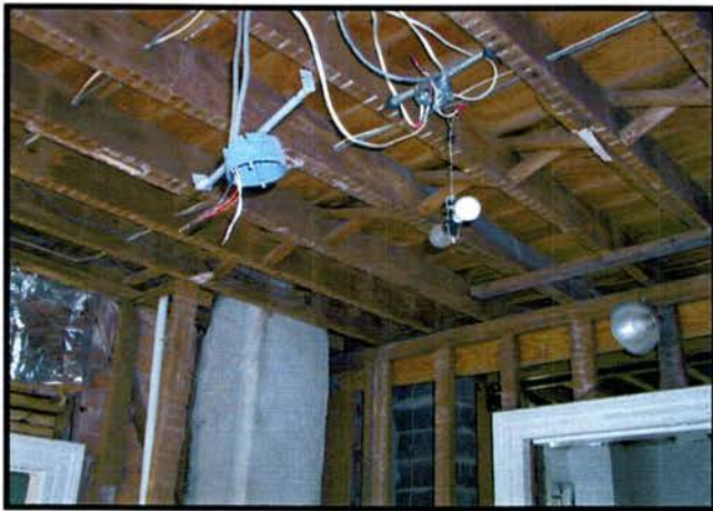
Left: ceiling in rear parlor, showing bridging and new electrical wiring as well as repairs to chimney and wall framing.
