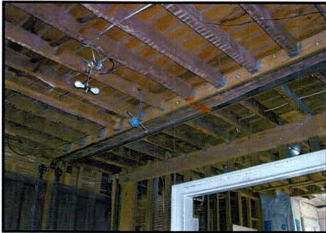
Left: ceiling framing in the front parlor, showing structural repairs made to existing floor joists and marks from old lath strips.
