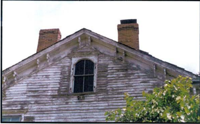
Peak of south gable shows brackets and arched attic window. Meadows Foundation volunteers made repairs to rotted cornice during the roofing campaign.
