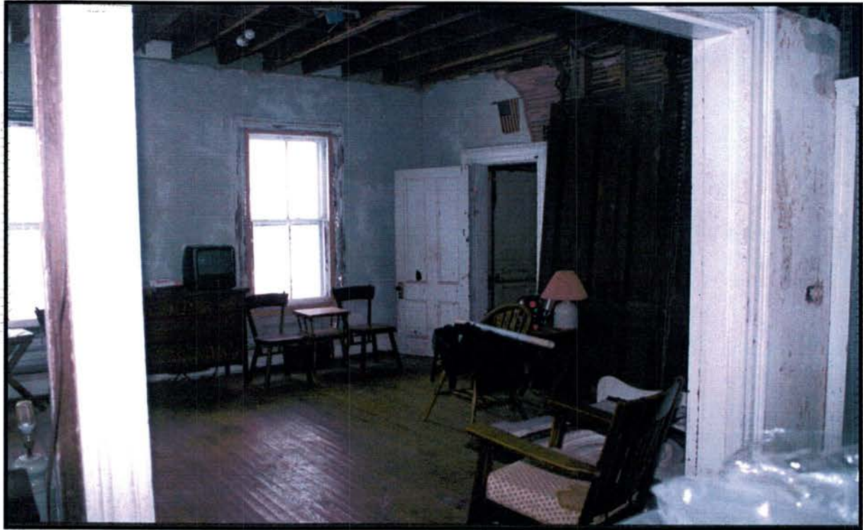
View of front parlor, 105, from rear parlor, 106, showing the open ceiling and partially stripped plaster walls.
