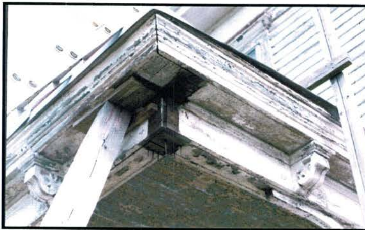
Below left: a detail of the cornice and architrave of the porch. Scroll brackets were placed at regular intervals in the architrave, with one between each post and one marking the post locations.
