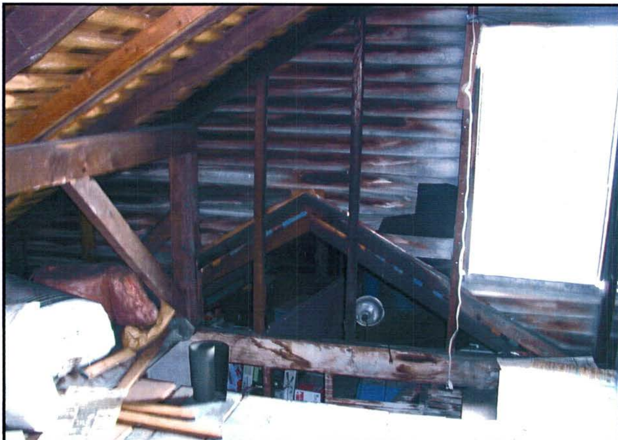
South wing attic, looking north toward roof join between the two builds. No evidence was found of a lower roofline at this juncture, but the current roof framing is exposed.
