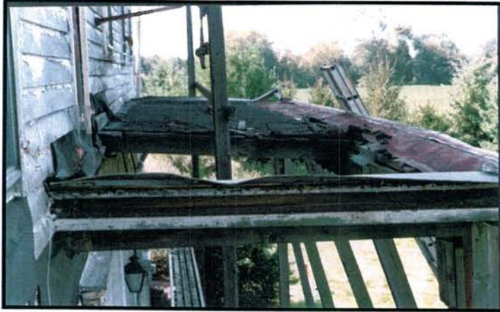
Above left: the collapsed roof of the porch and framing members. Note the metal at the right.
