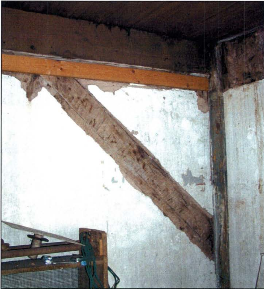
Room 100, view of corner post and diagonal brace at southwest corner. The upper board is a recent addition and will be removed.
