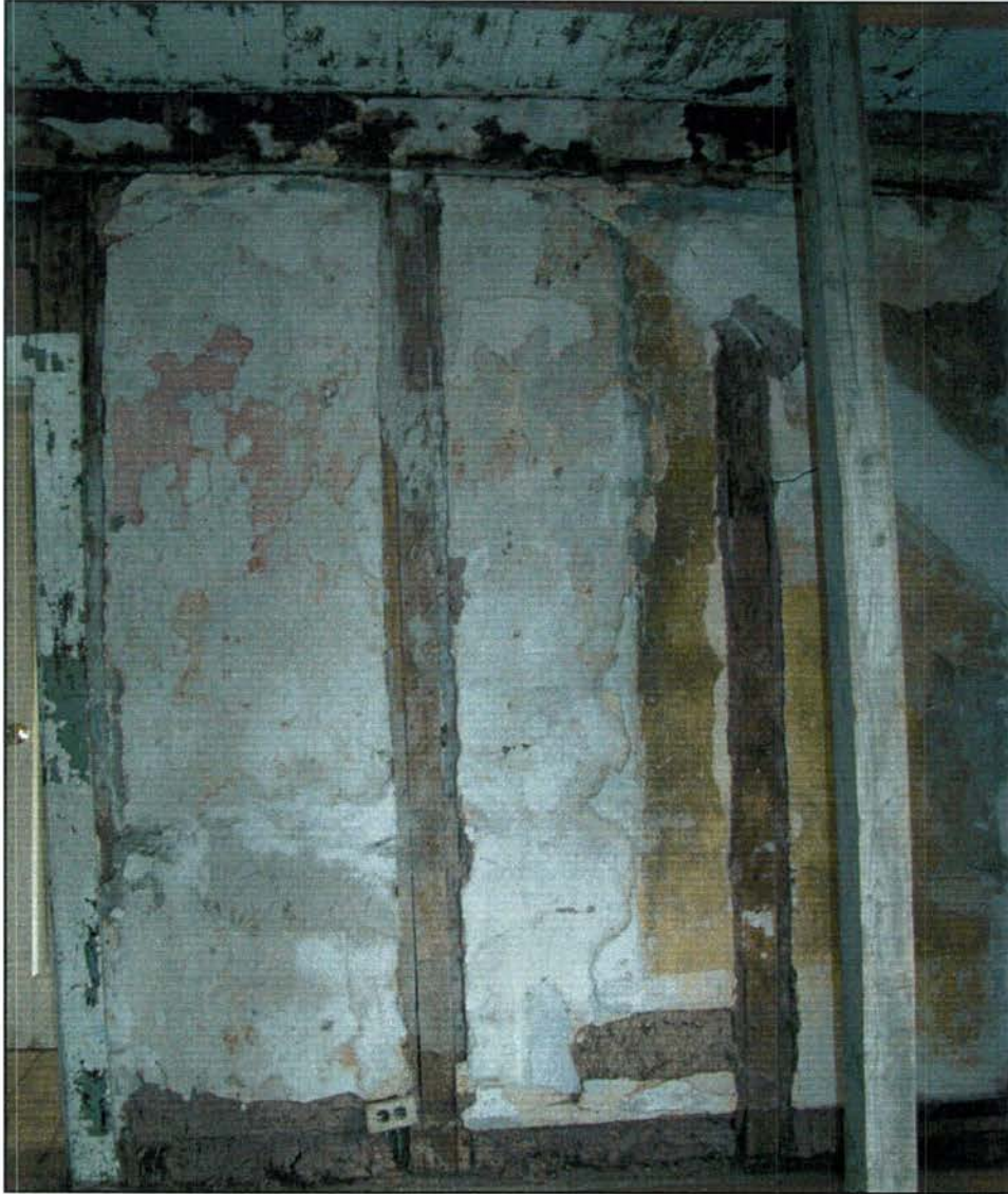
Room 102, south wall. Original plaster and studs reveal the construction methods and the sequence of the two builds.
