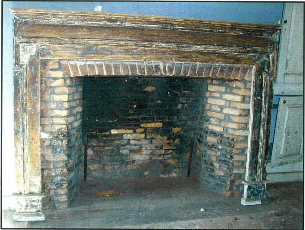
Room 103, fireplace opening and mantelpiece following the removal of sheetrock. The plaster line revealed that the mantel dates from construction of the English fireplace, c. 1750. The firebox post-dates the original build.
