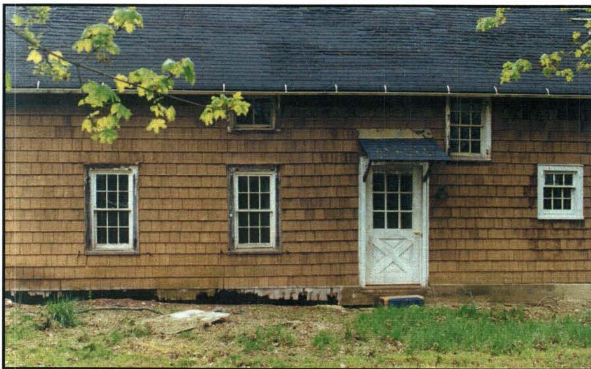
Perspective-corrected image of the northern portion of the west facade, showing early 19th century window openings from the Garretson build, in 1805.
