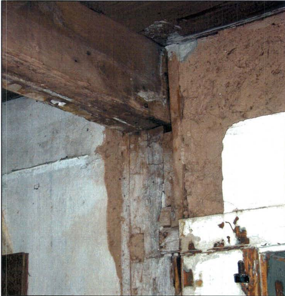
Room 100, detail of anchor beam and inner wall post adjoining Room 103. This wall retains its original finishes and construction details, including the door frame below right.
