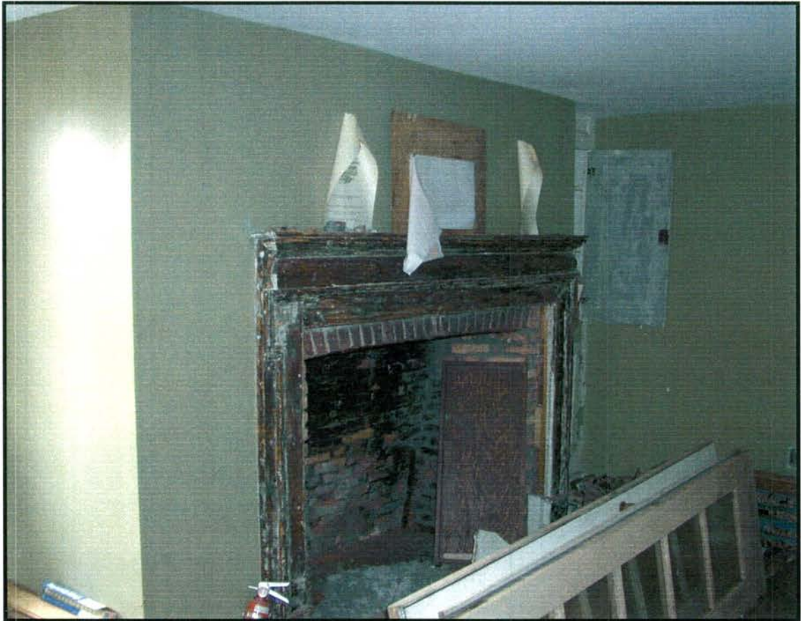
Room 103, Front chamber or “Groot Kammer,” before probes revealed the ceiling and chimney configuration.
