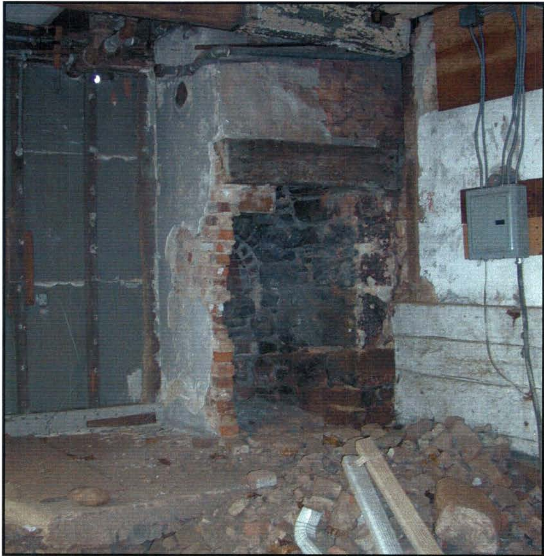
Room 102, former kitchen, looking north toward truncated cooking fireplace. The floor in this room was removed for foundation repairs ten years ago.
