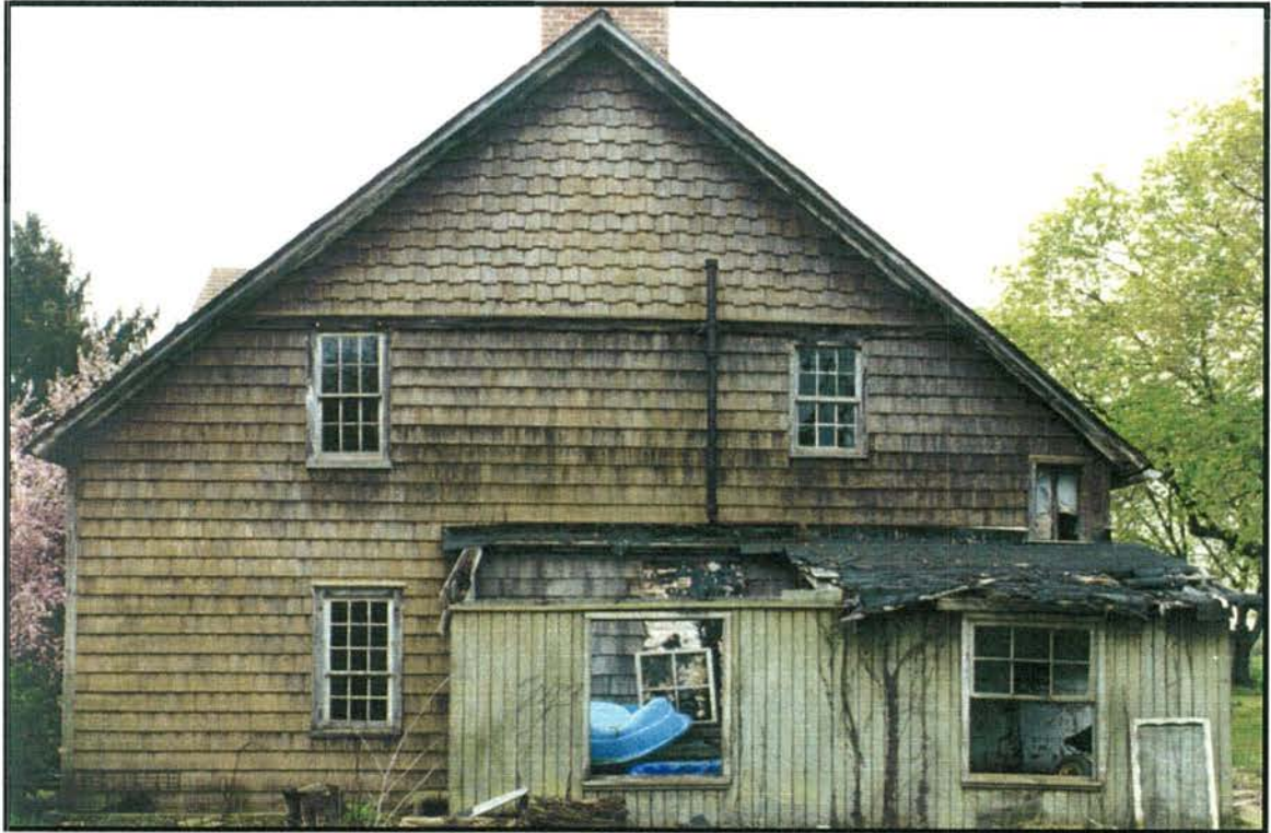
Perspective-corrected image of the north facade of the Wyckoff-Garretson house, before removal of the lean-to.
