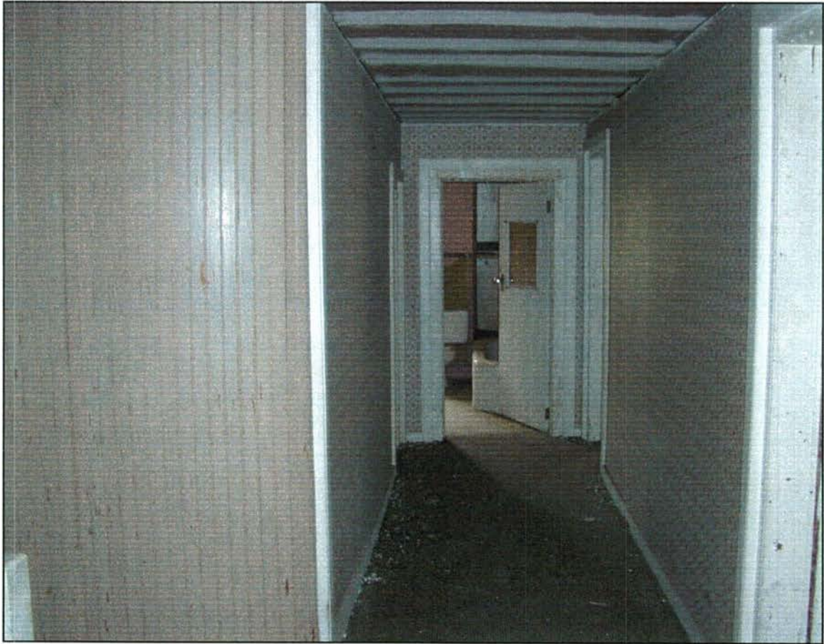
Room 201, upper stair hall, looking toward bathroom on north end of building.
