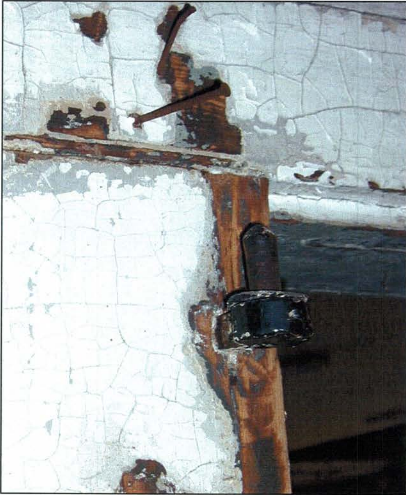
Room 100, detail of 18th century iron pintle used to hang the original door in opening No. 6. The nail above is a cut nail. The original finish is the Venetian red found in the trim of the first build.
