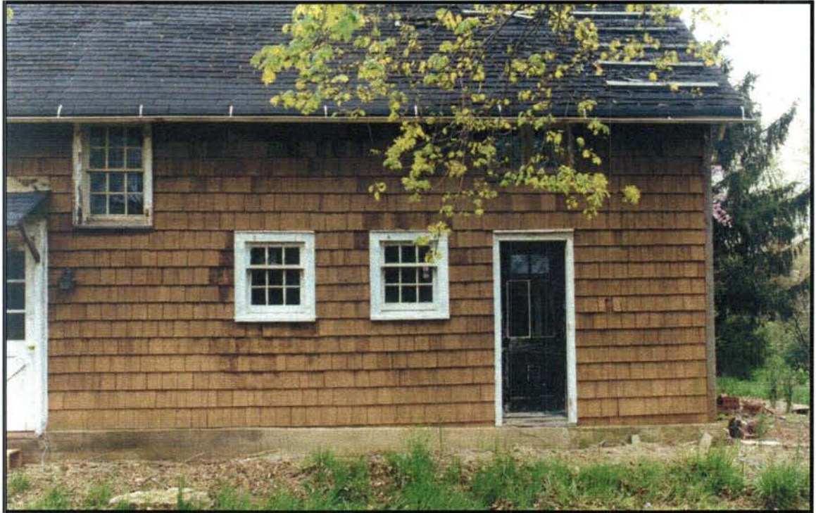
Perspective-corrected image of southern half of west facade, showing the portion of the house constructed by John Wyckoff. All of the openings have been changed since the early 19th century.
