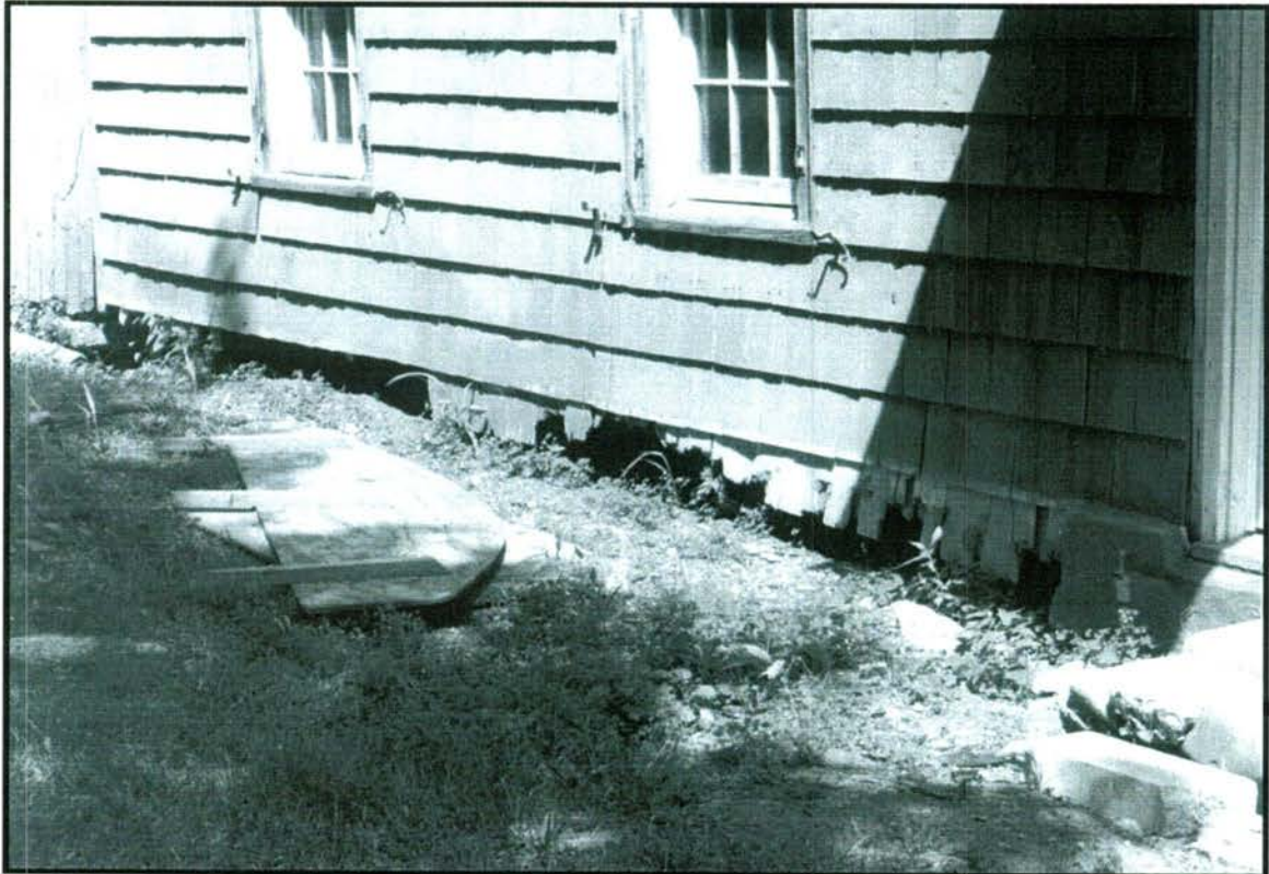
Close-up view of missing sill, foundation wall damage, and rotted shingles at base of west wall.
